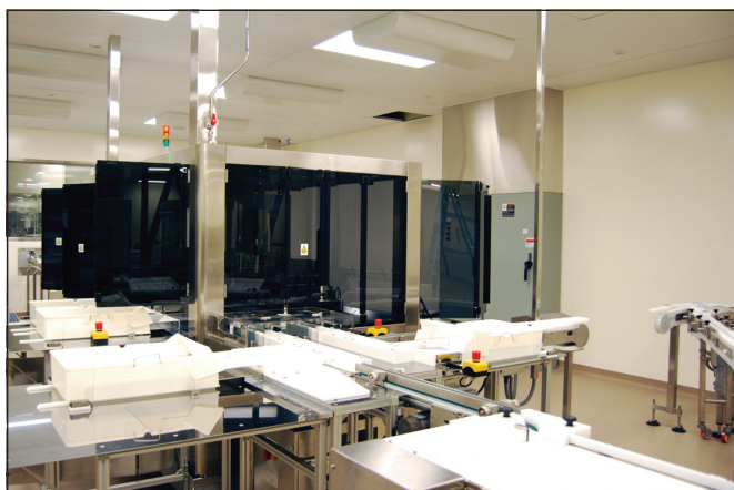
Figure 5. Inspection lines are visually connected to the fill suites to ensure ease of communication. Within the inspection suite, there is the capability for both automated and manual inspection.
