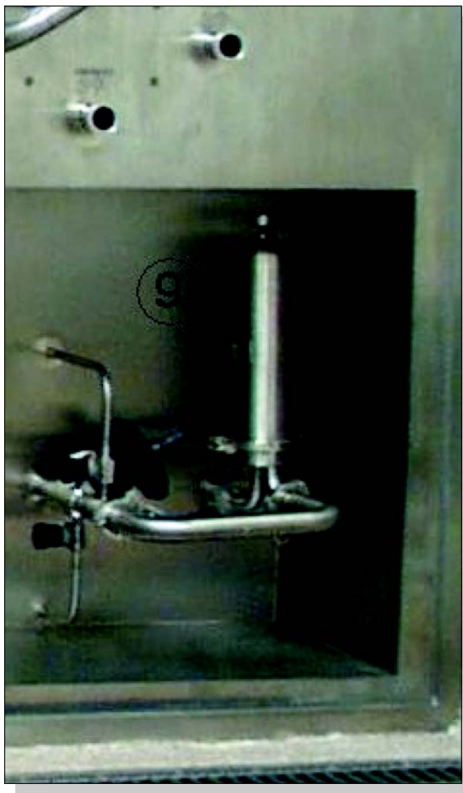
Figure 5. Transfer panel integral filters.
